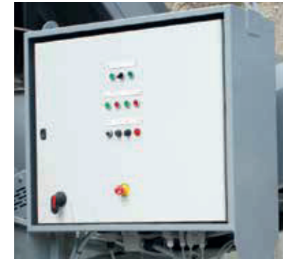
H12 Feeder Control Panel
