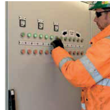
Central control panel for typical large washplant installation
