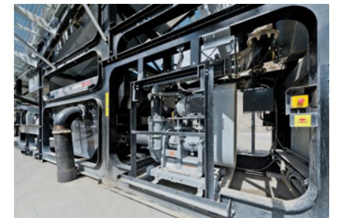
Centrifugal Pumps, Roll out for Service Access
